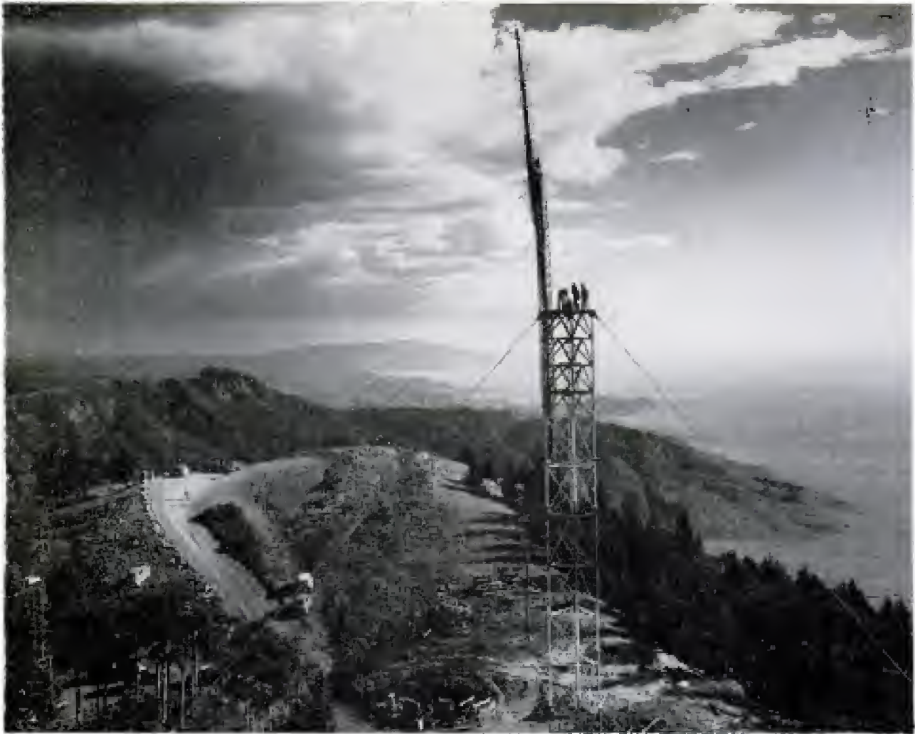
Workmen install antenna of KGGM-TV on edge of mountain. Mesa 5000 feet below is at the Albuquerque level
